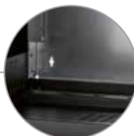
Omega-type reinforcement and cable fixing for an orderly cabling
